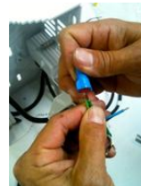
Using provided waterproof wire nuts, mate three corresponding wires to step down power supply input wiring
