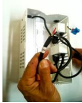
Locate 12VDC Cable from power supply output, this go into D2 enclosure
