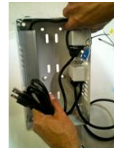
Tighten Strain relief nut around wire just installed, then Re-install plastic box onto Metal Bracket using original fasteners.
