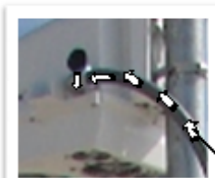
Arrows illustrate air flow within conduit when wire feed is not sealed within enclosure
